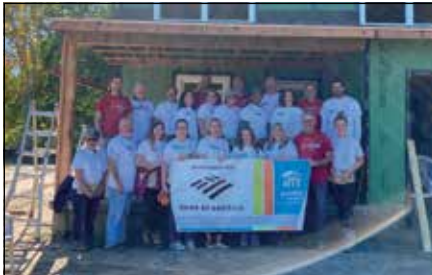
Bank of America teammates took a break from roofing and siding at Habitat for Humanity site during annual Global Build Week.
